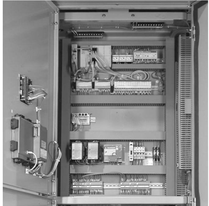
Master Control Section Interior
